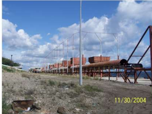
Plant wharf receiving unit
